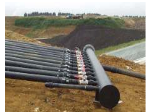
Landfill Gas Recovery
