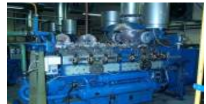
Cogeneration produces electrical power and captures waste heat with high efficiencies
