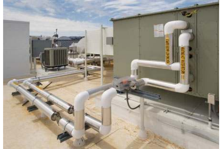
Building HVAC Systems Can Be Optimized
