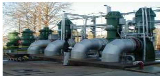
Pumps & Motors Can Be a Source of Savings
