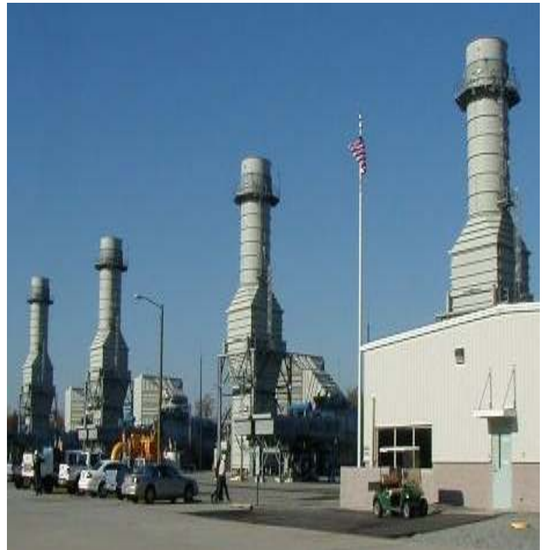
Combine-Cycle CHP Cogeneration System
